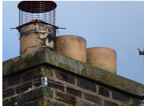
Cracked chimney pot/open pots
