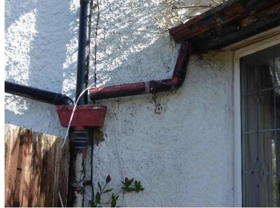
Leaking rainwater pipes
