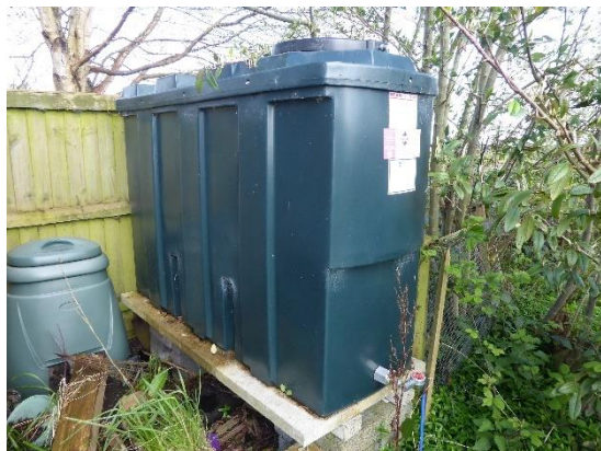
Oil storage tank
