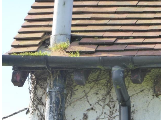
Tile repairs required
