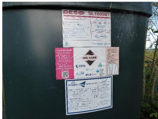
Oil storage tank
