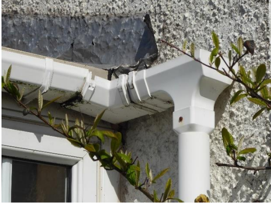
Loose rainwater fittings
