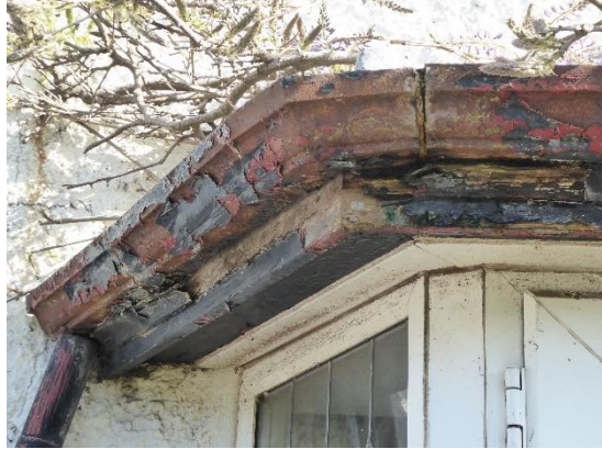
Corroded/leaking cast-iron gutters
