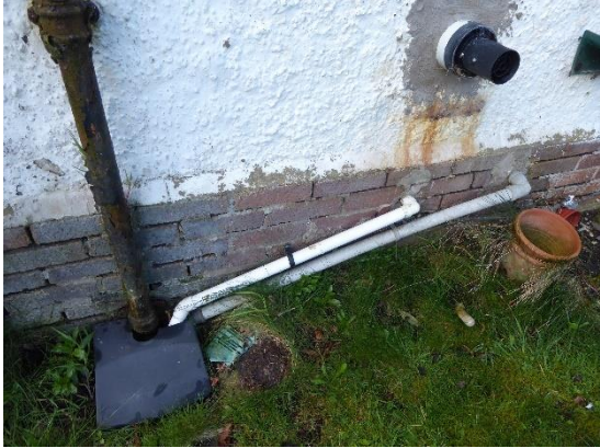
Kitchen waste pipes
