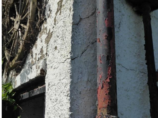
Cracking to rear corner
