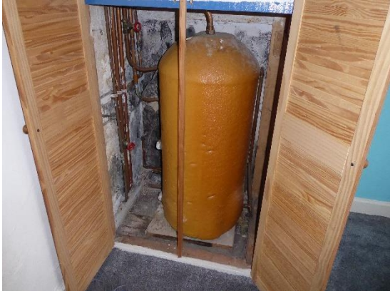
Hot water cylinder
