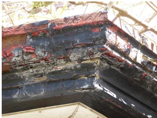
Evidence of decay
