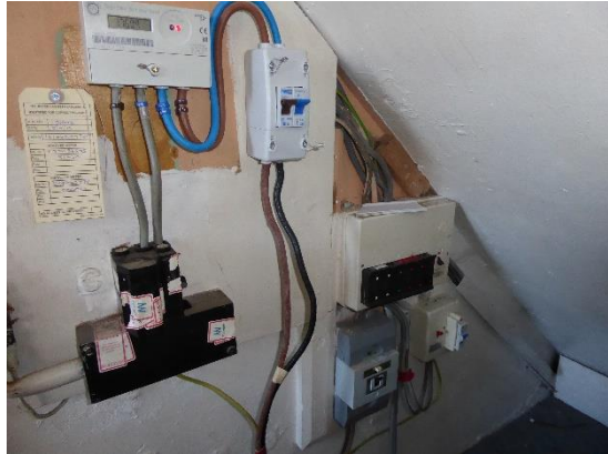
Electric meter and consumer unit (fuseboard)
