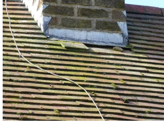
Tile repairs required
