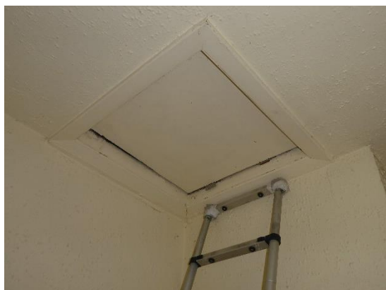
Loft hatch – sealed/jammed shut
