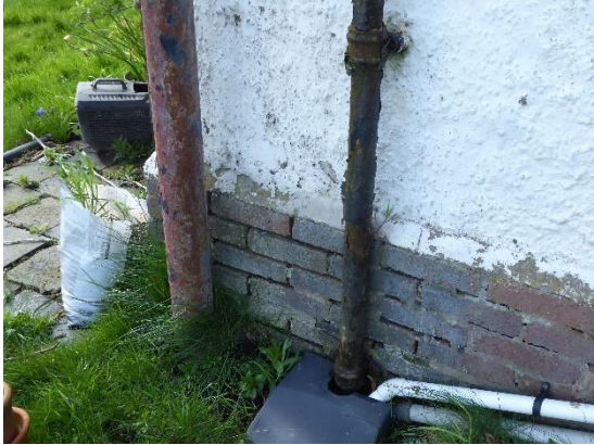
Corrosion to cast-iron sections
