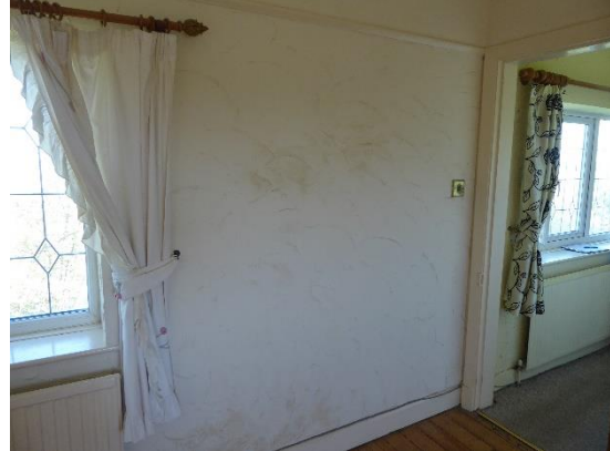
Internal cracking to landing area
