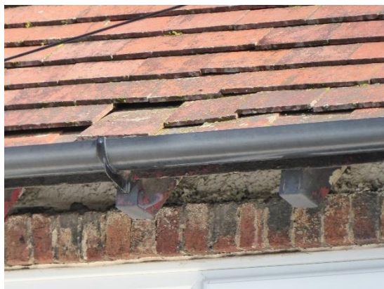
Tile repairs required
