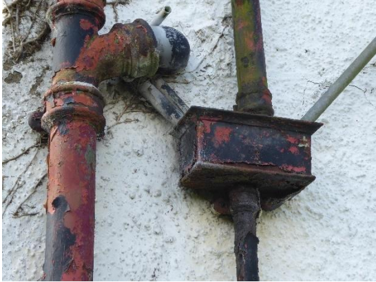
Corrosion to cast-iron sections
