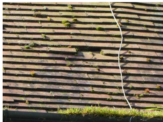
Tile repairs required
