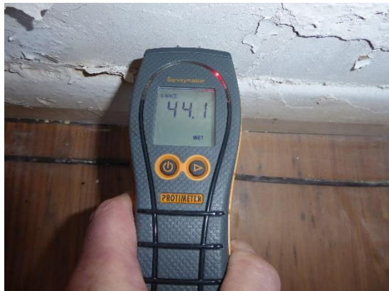
Evidence of dampness within the ground floor walls
