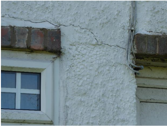
Cracking above window/door openings
