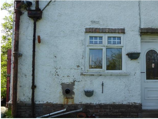
Cracking to rear corner
