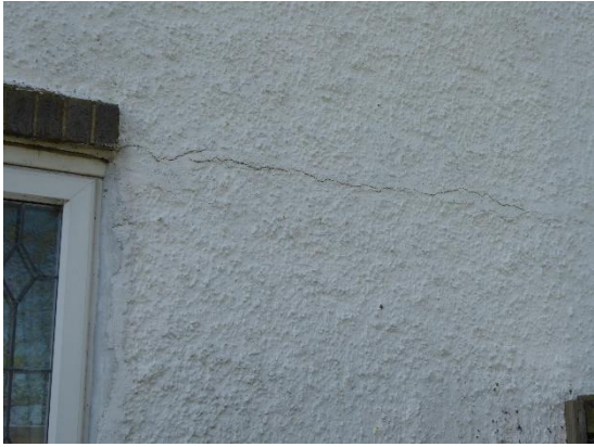
Cracking above window/door openings
