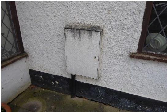
Electric meter location
