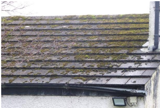
Out of level/loose gutter to rear extension
