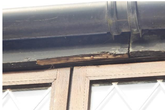
Evidence of decay
