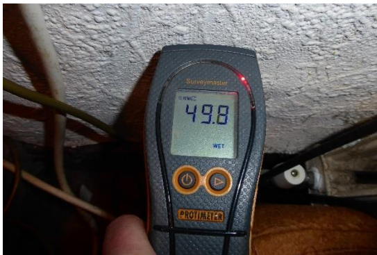
High moisture meter readings to the ground floor walls
