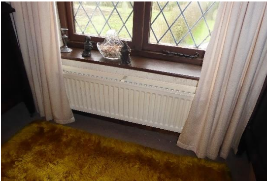
Safety concern – no safety glass
