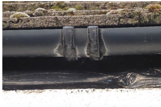
Leaking gutter joints
