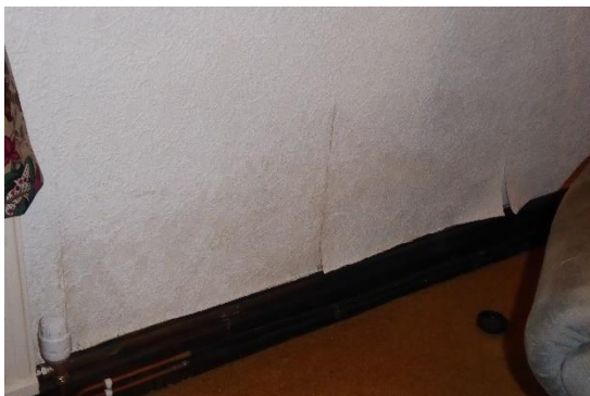
Damp staining to ground floor walls
