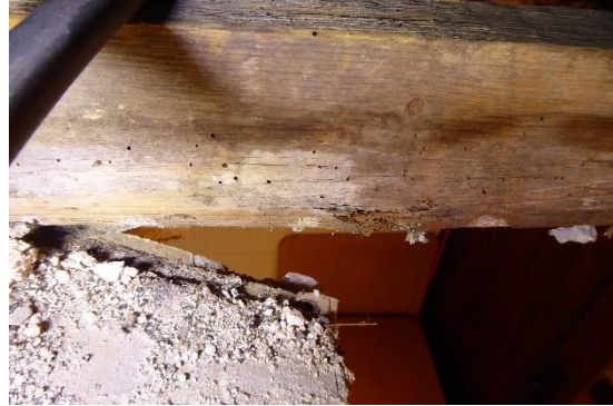
Evidence of wood woodworm infestation
