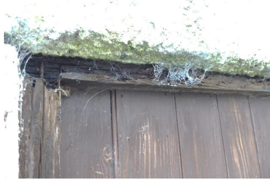
Decay to door frame
