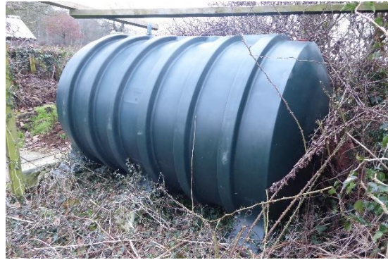
Oil storage tank
