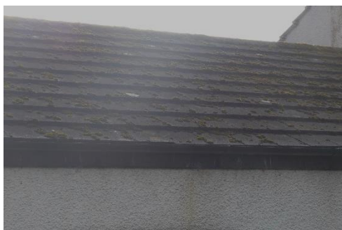
Moss on roof coverings
