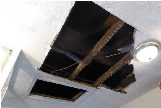
Water damaged Bathroom ceiling
