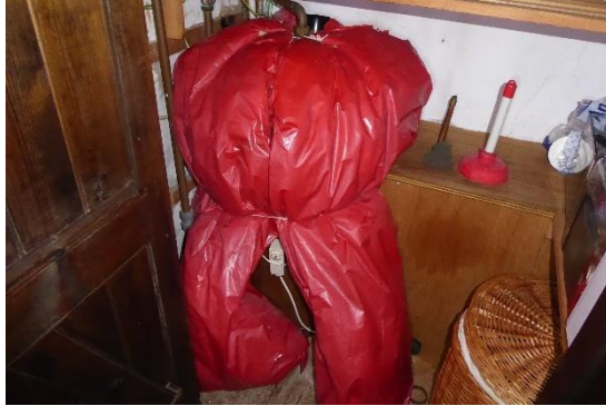
Hot water cylinder
