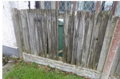
Decayed boundary fencing
