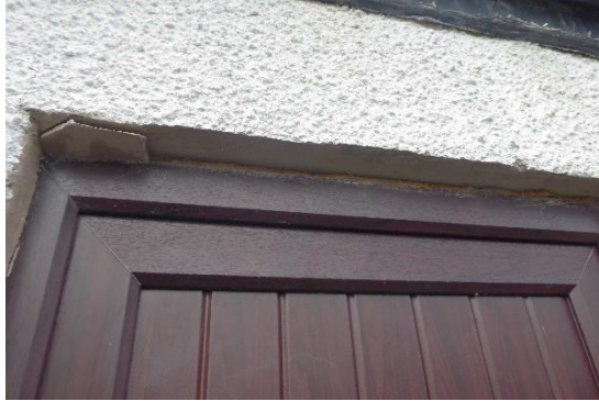
Front door – missing frame sealants
