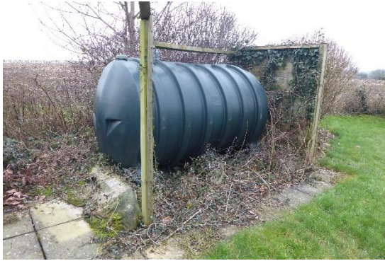
Oil storage tank
