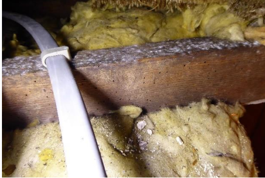
Evidence of wood woodworm infestation
