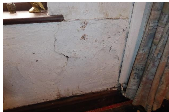
Textured finishes that may contain asbestos fibres
