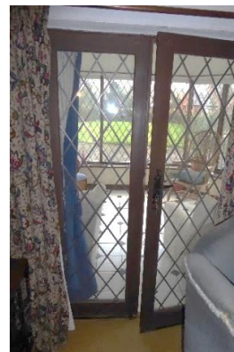
Safety concern – no safety glass
